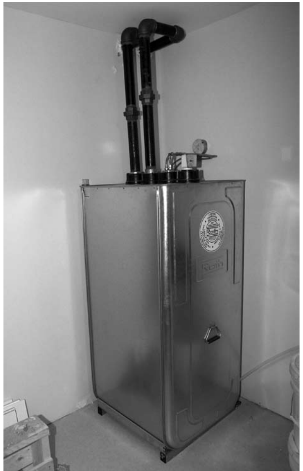
Double walled oil tank with two pipe fuel line system exiting the top of the tank.
