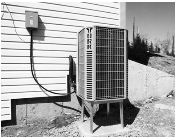
Air-to-air heat pump – exterior unit.
