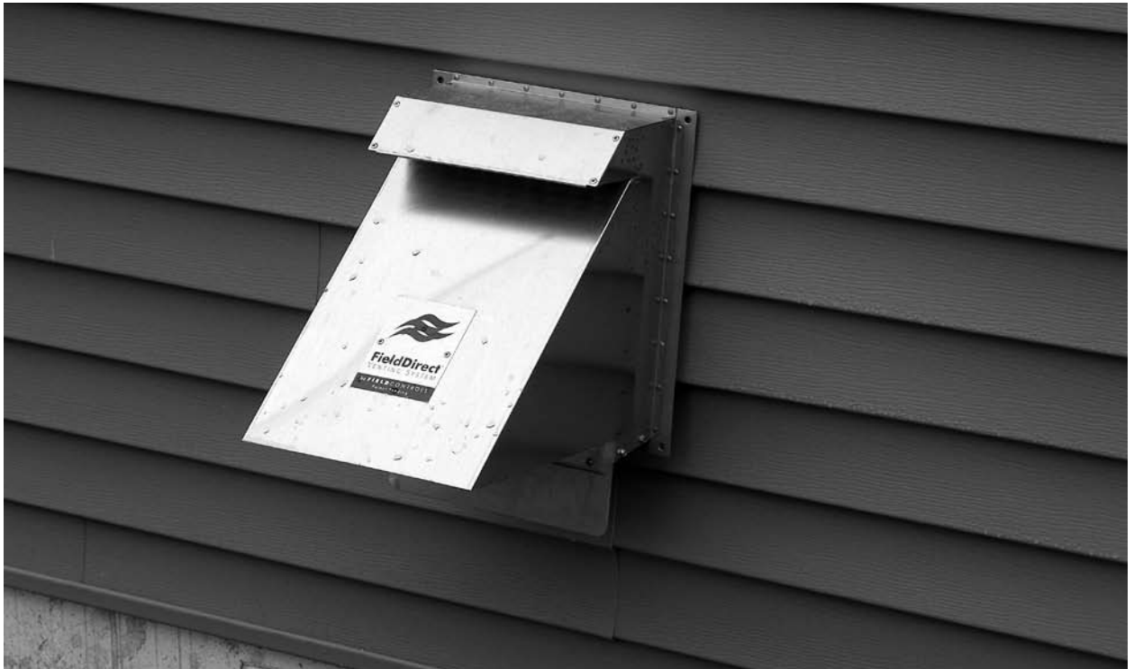
Exterior direct-vent exhaust hood.
