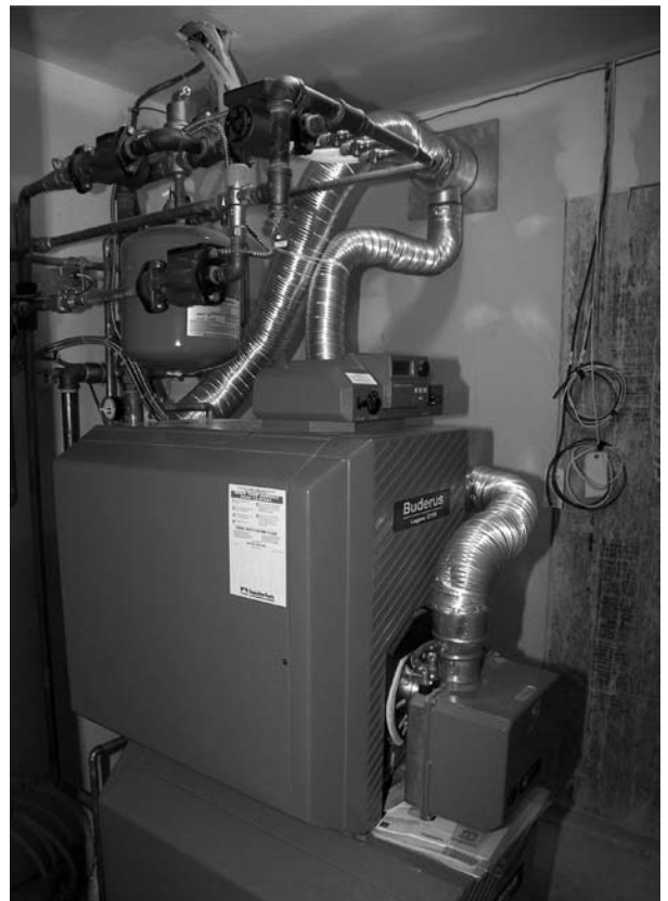
Direct-vented oil-fired boiler. The domestic hot water tank is under the boiler/burner.
